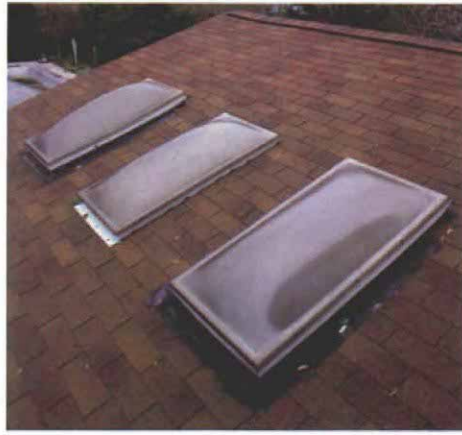
Curb-flashed skylights rely on a mastic seal. When the mastic seal around these curb-flashed skylights failed, roof cement was incorrectly applied on the shingles to stop a leak.
