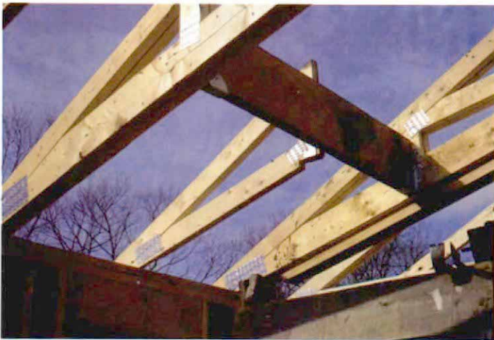
Wide skylights in truss roofs. A truss roof can be engineered to accept a wide skylight. Here, trusses have been doubled, and a small monotruss that fills in the roof below the skylight hangs on a header.
