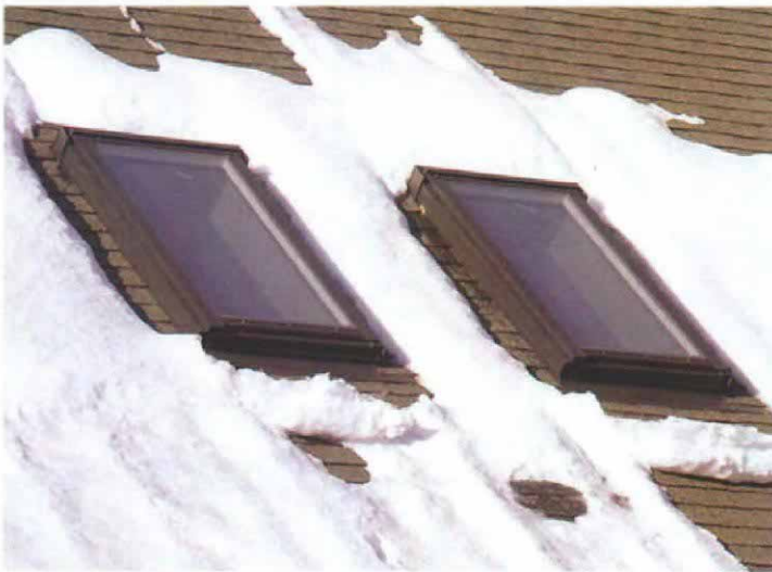
Bare shingles can indicate air leakage. Step-flashed skylights have to be sealed with felt paper under the flashing to make them airtight. If not done properly or skipped altogether, warm air leaking from inside will melt the snow around the perimeter of the skylight.
